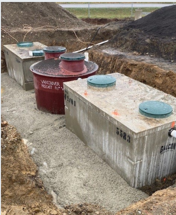
Septic system – Feb 21st
