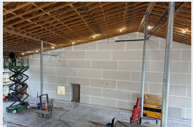
Apparatus Bay E&W walls taped
