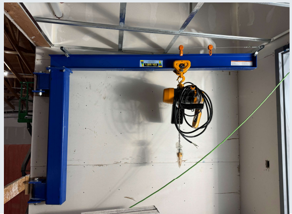
Jib crane mounted
