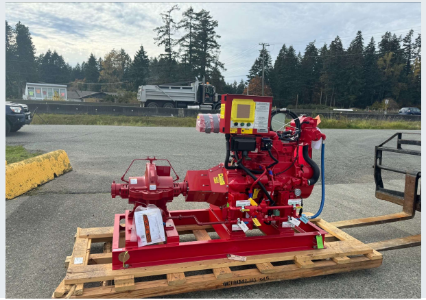
Fire pump delivered
